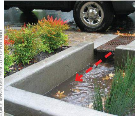
Figure 5-19: A grated curb cut allows stormwater to pass under a pedestrian egress zone to the stormwater facility.
