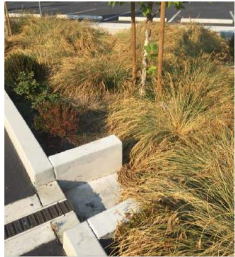
Figure 5-13: The side wings and concrete apron of this trench drain curb cut prevent blockage & erosion. (Credit EOA, Inc.)
