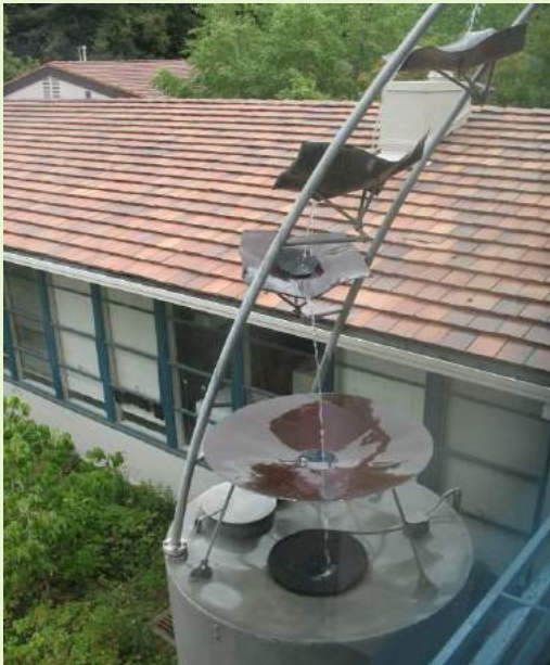
Figure 6-48: Rainwater is collected and used for flushing toilets at Mills College, Oakland. (Credit: EOA, Inc.)
