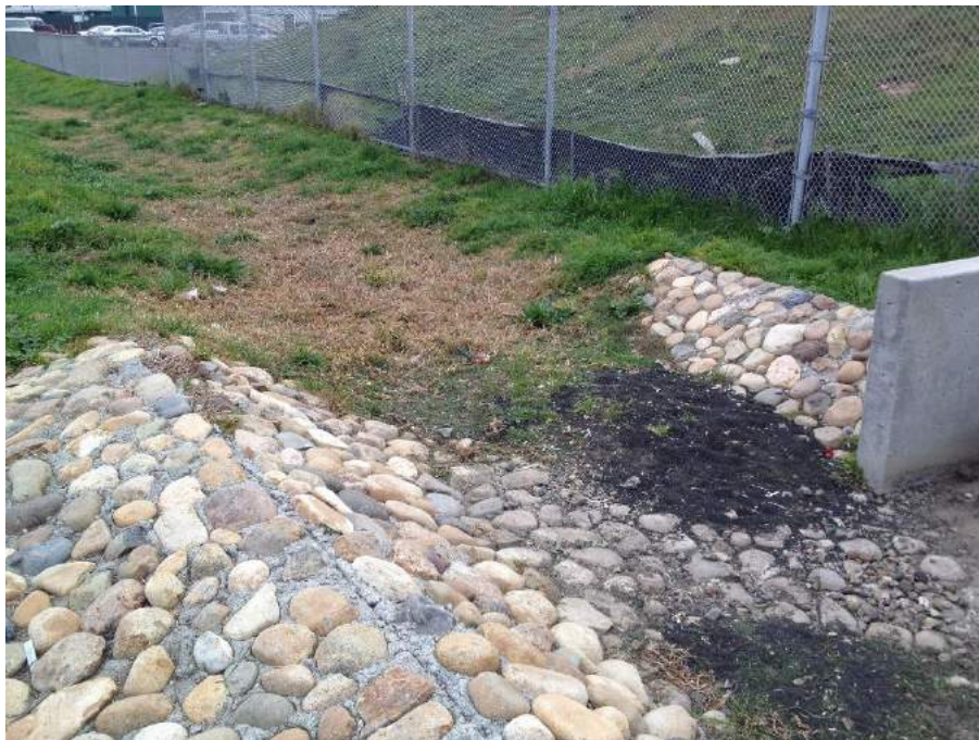
Figure 5-7: This bioretention area treats runoff from an artificial turf field in Berkeley and has an accumulation of crumb rubber particles (the black areas in the photo). (Credit: EOA, Inc.)
