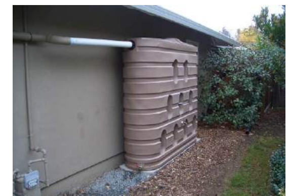
Large unit installed at a single family residence. Courtesy of Stephanie Morris
