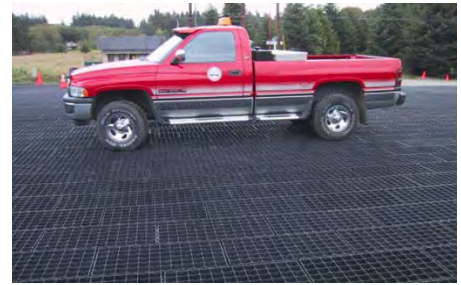
New installation of reinforced grass pavement. Photo: Puget Sound Action Team, WA
