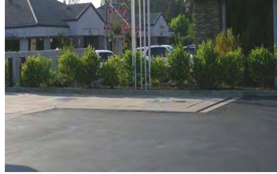
This retail gasoline outlet in Folsom has perimeter drains around both the concrete fueling pad and the concrete fuel transfer area. The drain carries spills and runoff to an onsite underground containment tank.
