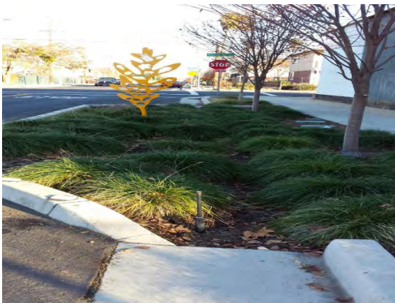
Dixie Ave Bioretention Planter, City of Sacramento
