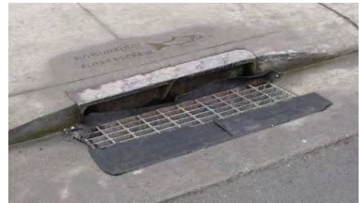
Inlet marking directly in concrete Photo source: County of Sacramento
