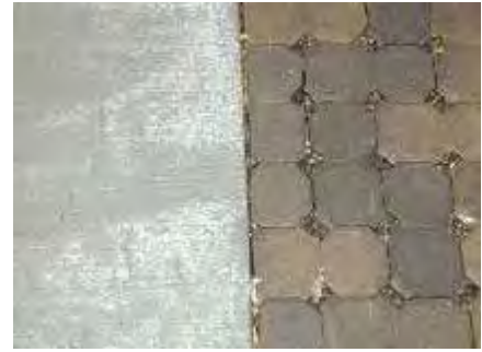
A water barrier or interceptor drain will be required between regular load-bearing pavement/streets and porous pavement materials. Photo: City of Portland
