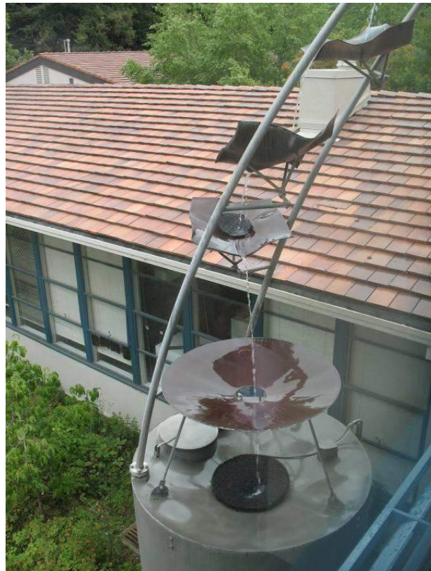
Photo 8-8. Rainwater harvesting system, Mills College, Oakland
