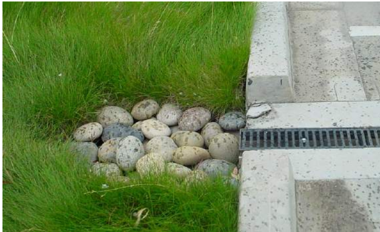
Photo 5-3. Cobbles are placed at the inlet to this stormwater treatment measure in Fremont, to help prevent erosion.
