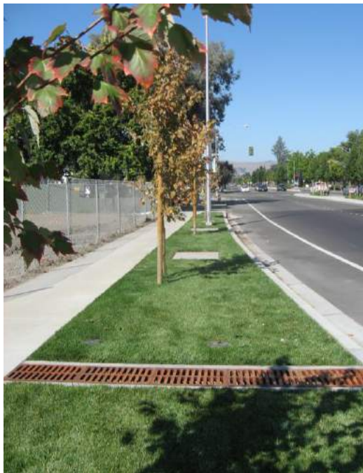
Photo 8-3. Series of non-proprietary tree well filters installed along roadway, City of Fremont
