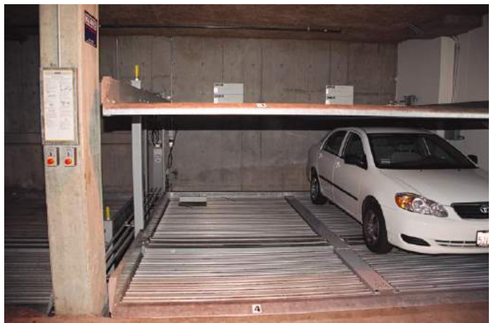
Photo 4-1. Parking Lifts in Parking Garage, Berkeley
