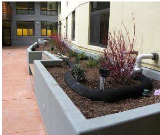
Photo 6.2-2. Half-buried, perforated flexible pipe serves as a flow spreader to distribute stormwater evenly throughout long, linear flow-through planter in Emeryville
