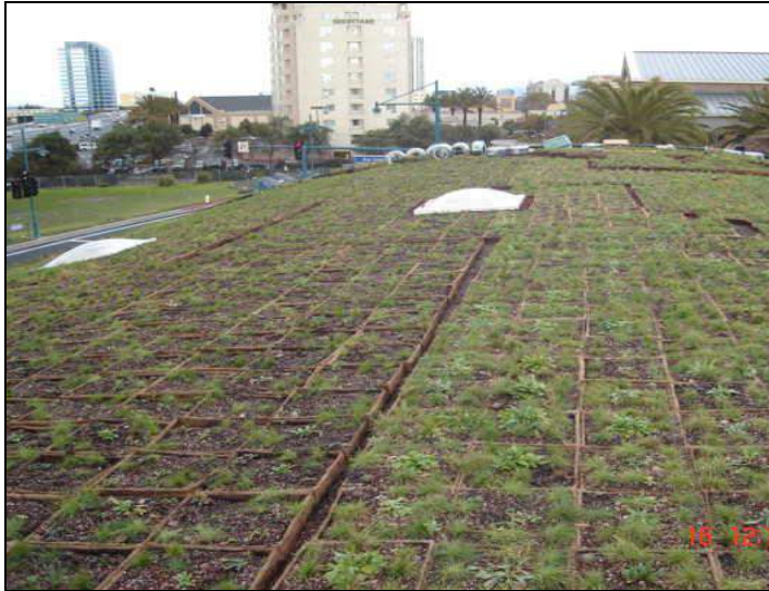
Photo 6.8-1. Extensive Green Roof in Emeryville
