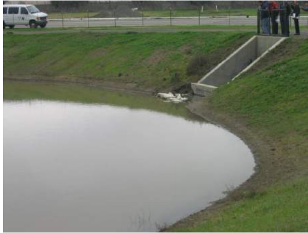
Photo 5-2. Detention pond in Pleasanton provides hydromodification management.
